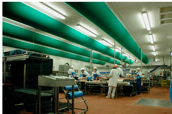
Process cooling: Dalehead Foods, Bury St. Edmunds, UK
