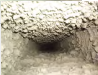
” A clean ventilation duct and a duct with deposits of dust and dirt. ”
