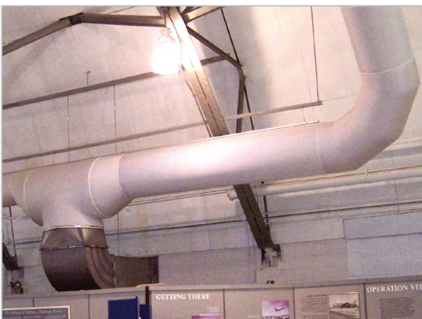
Sample installation: T-piece with a conical transition (flat edge on top) and 90° bend running upwards
