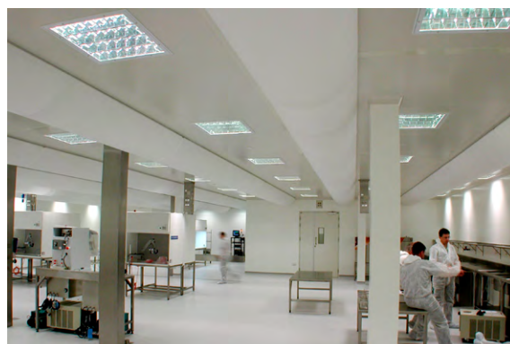
Clean room facility: Alcon Ireland, Ireland
